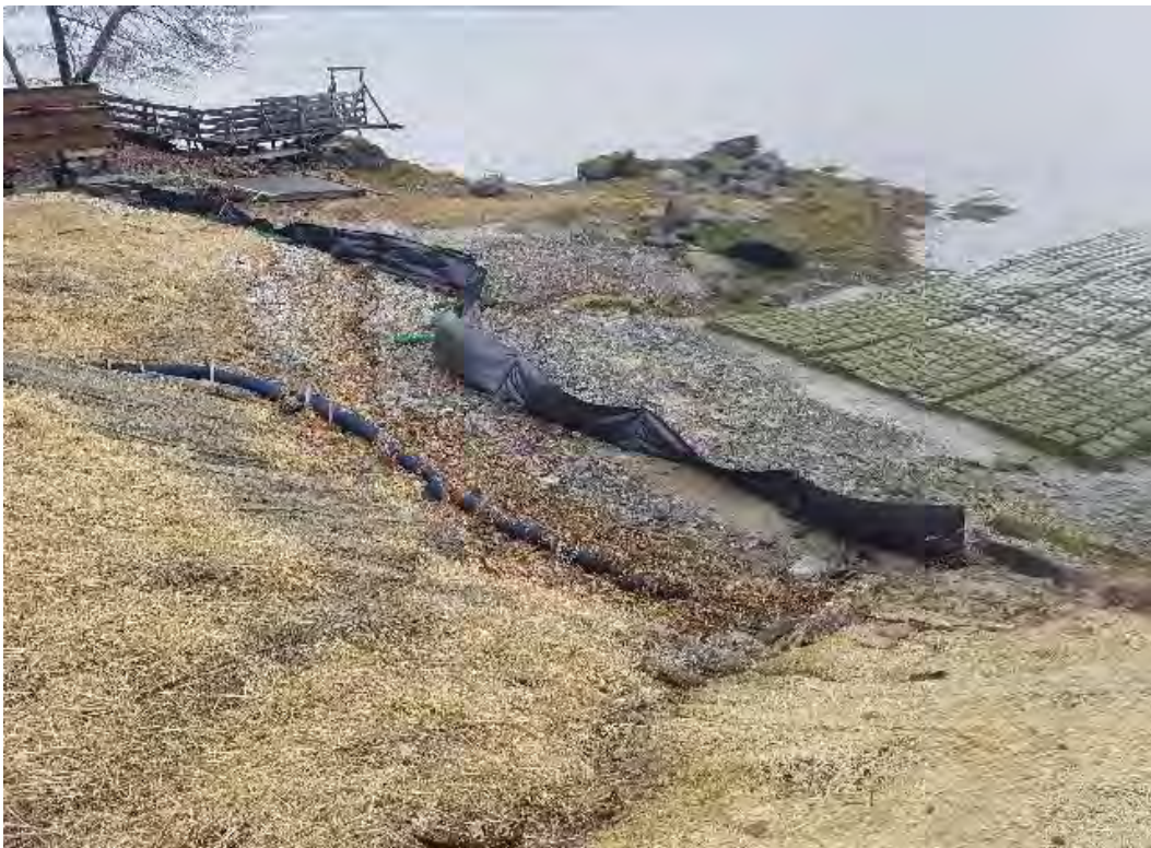
Fig 16: BMPs at toe of slope at Getchell property/west side of the Bay. Viewing northeast. (03-30-20).
