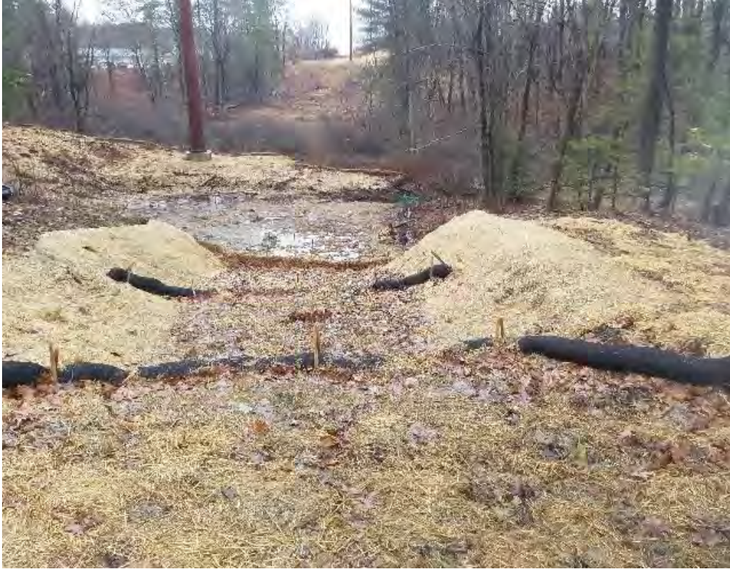
Fig 11: Access road to Str. 28 and wetland DW49. See comments above. Viewing north. (03-30-20).
