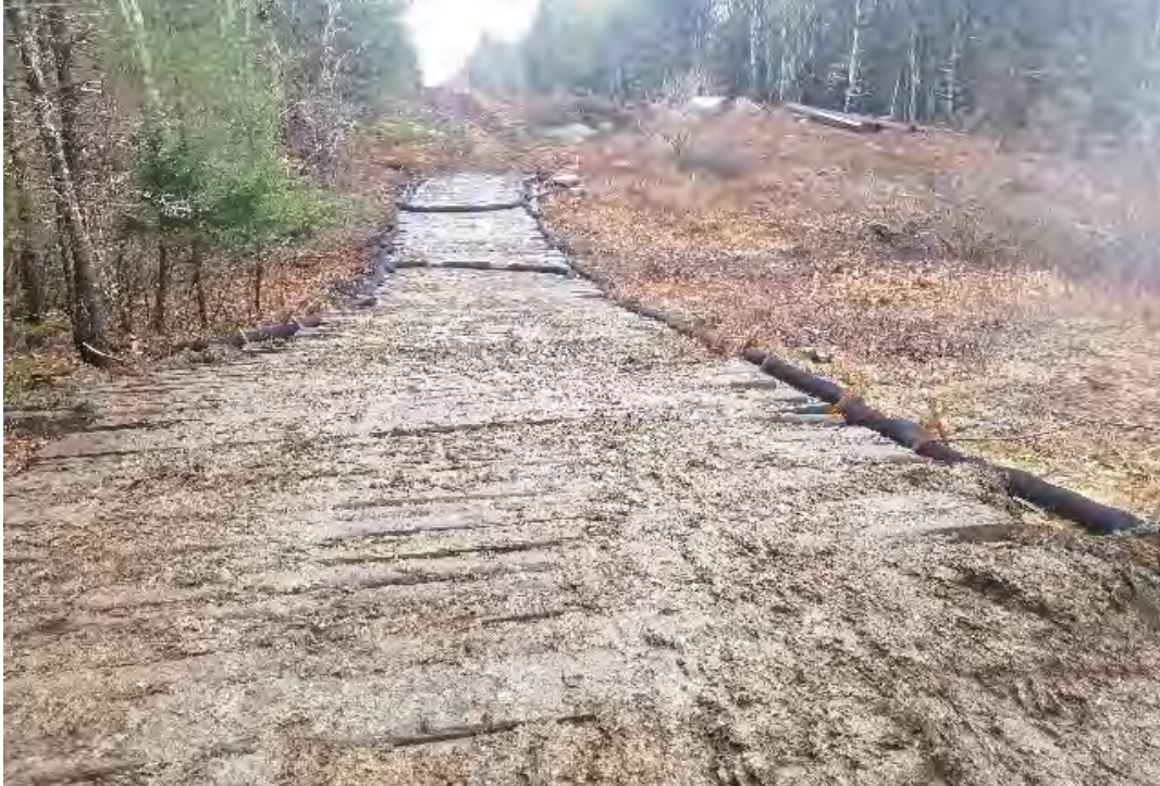
Fig 13: Access road between Strs. 85 and 84, through wetland DW30 and over stream DS32. Viewing west. (03-30-20).
