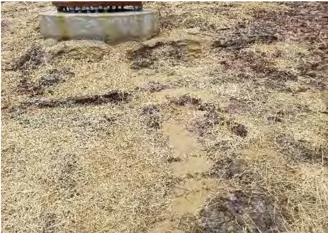
Fig 12: Erosion at Str. 29 foundation. See comments above. Viewing south. (03-30-20).
