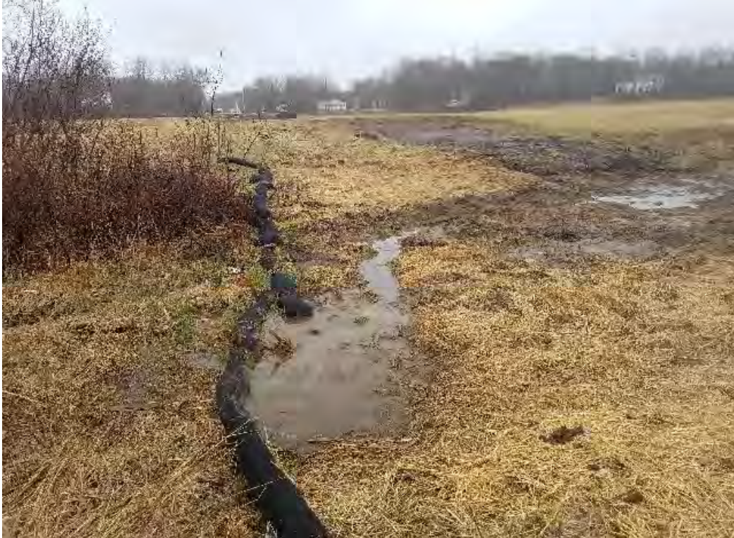
Fig 5: Erosion in wetland NW18 at Frink farm. See comments above. Viewing east. (03-30-20).
